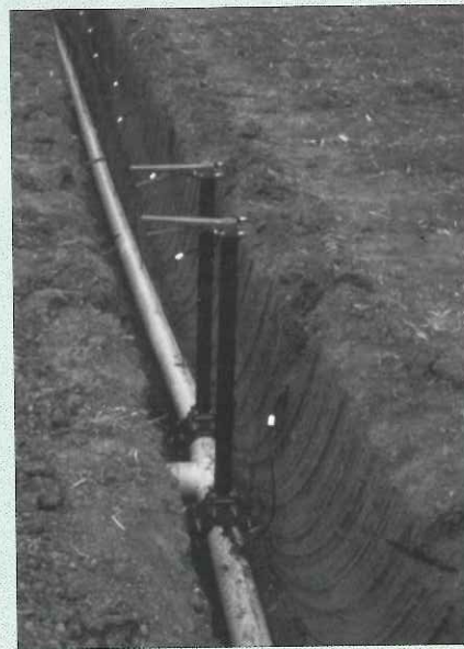
Installation showing main line and emitter tapes. The two handles are used to change the flow of water between the two irrigation sets.
