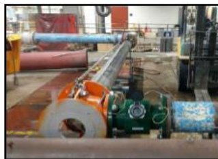
Zero Distance from Turbine Pump Discharge
