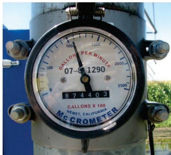
Figure J-2. Impeller flow meter commonly used to monitor the water flow rate in an irrigation pipeline.
