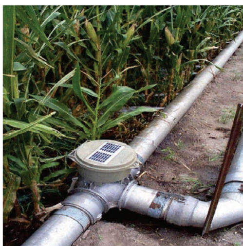
Figure K-5. Typical surge valve installation in the Platte Valley of Nebraska.
